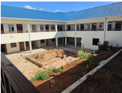
A team from Salt Lake will be planting the terraced gardens of the OPD courtyard. The gazebo is going up at the lower level.
