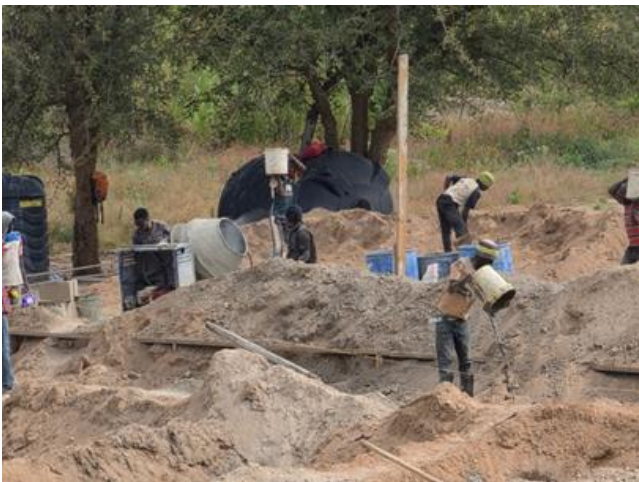
Work on the RCH is underway! All the work is being done manually!
